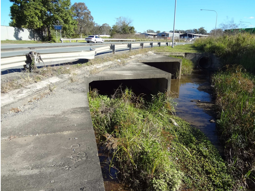
Oxley Creek Tributary – downstream side of the culvert (photo taken on the left culvert)
