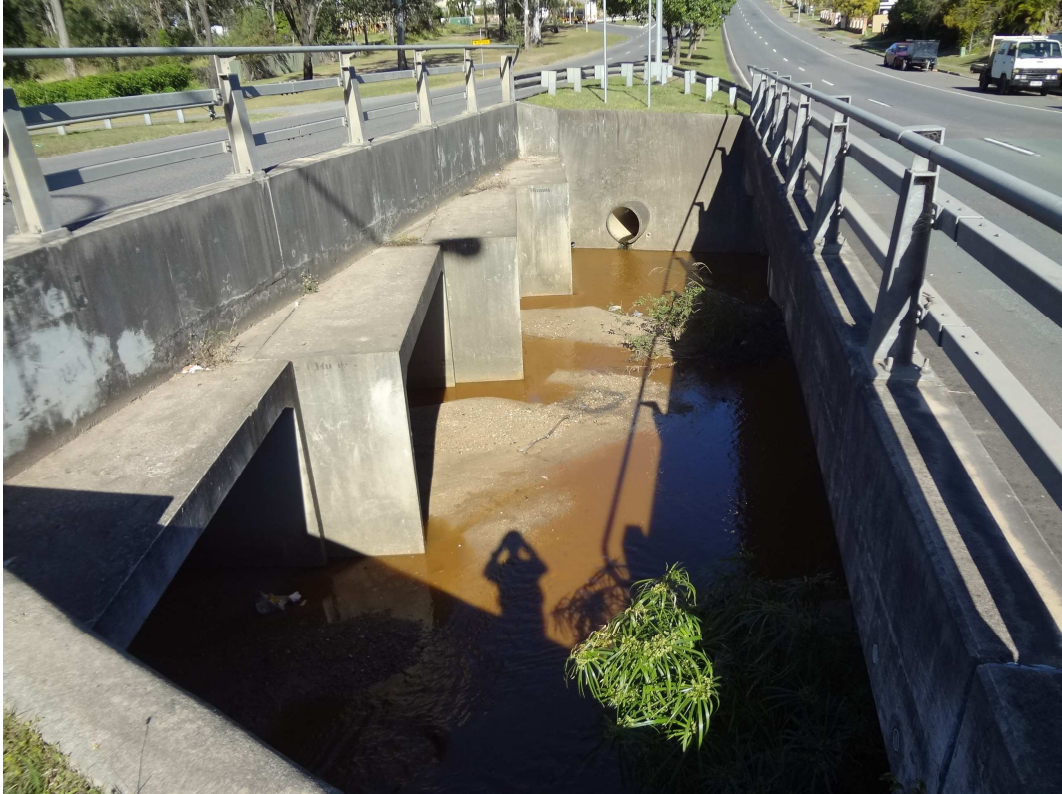
Blunder Creek Tributary – downstream side of the bridge and upstream side of the culvert
