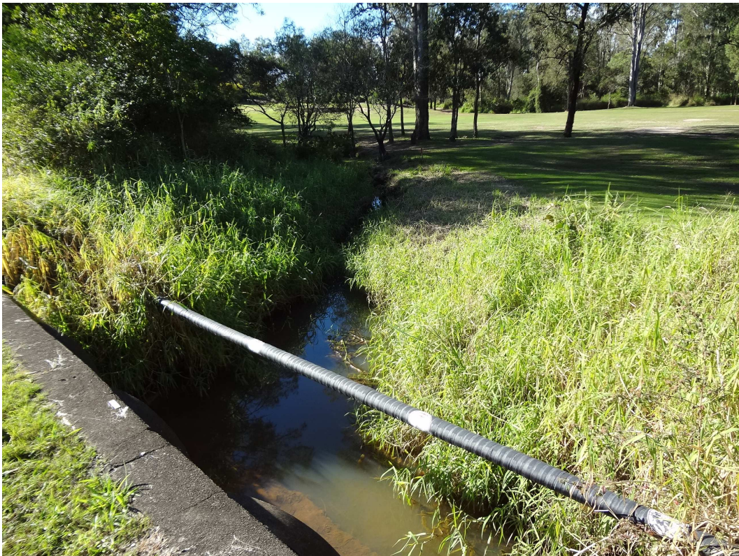
Oxley Creek Tributary – stand on the culvert looking downstream
